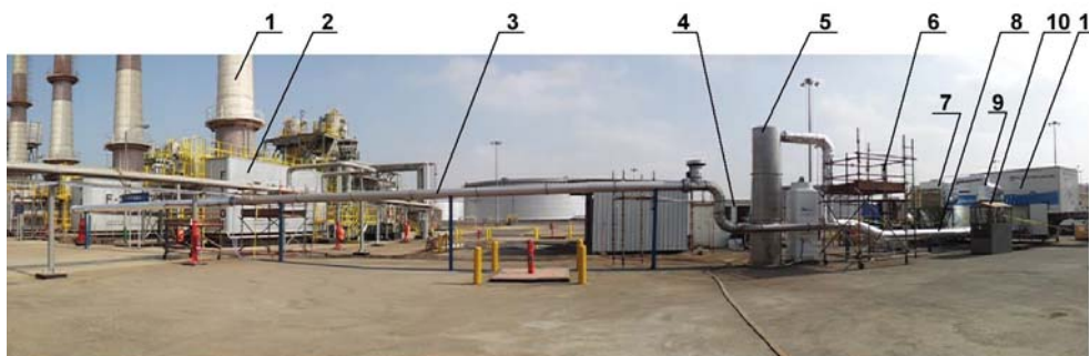
Fig.5. Pilot plant at oil refinery: 1 – stack of F 1001 boiler, 2 – boiler F 1001, 3 – flue gas duct, 4 – pilot plant control room, 5 – gas conditioning column, 6 – pilot plant stack, 7 – cartridge bag filter, 8 – thermal insulated duct, 9 – cyclone, 10 – ammonia dosing unit, 11 – mobile accelerator unit.
