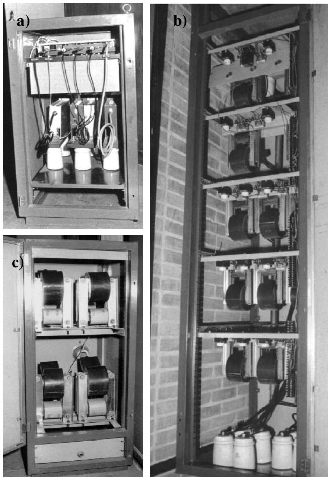
Fig. 2. Some parts of the galvanic separation barrier: (a) The optical fiber cable assemblies; (b) 24 VA high voltage low stray capacitance separation transformers; (c) 500 VA high voltage low stray capacitance separation transformers.
